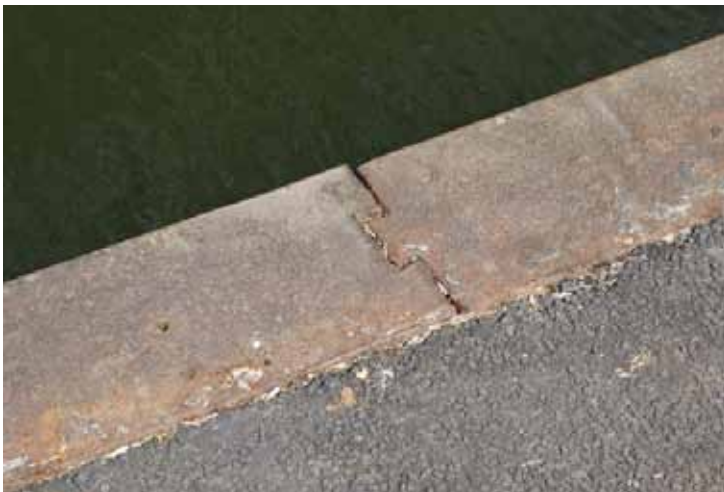
Cast iron reinforcing plates at the canal edge Rory Walsh © RGS-IBG Discovering Britain
