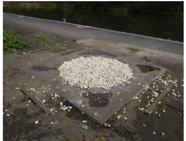
The metal crane base by the towpath Rory Walsh © RGS-IBG Discovering Britain
